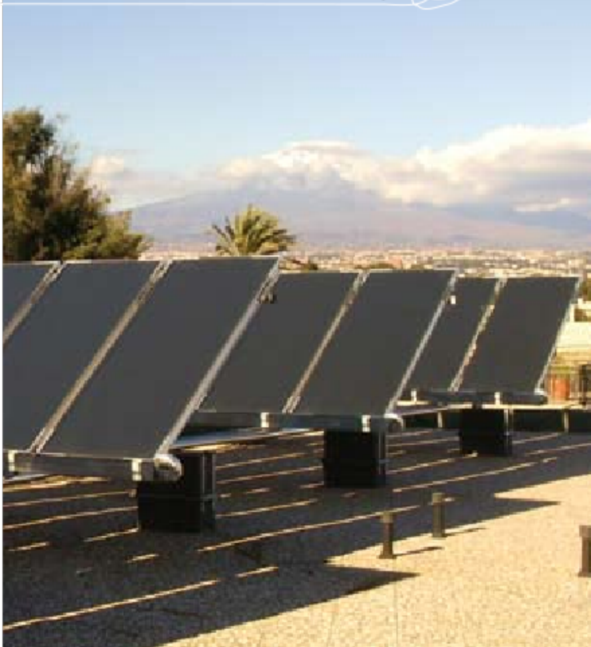
Solar panels at NH Parco degli Aragonesi Catania - Italy
